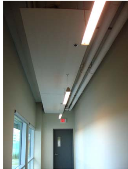
Figure 3: Radiant cooling panel in CDC (daylighting controls commissioning still in progress)
